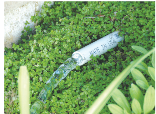
Figure 5 - System Rinse Line
